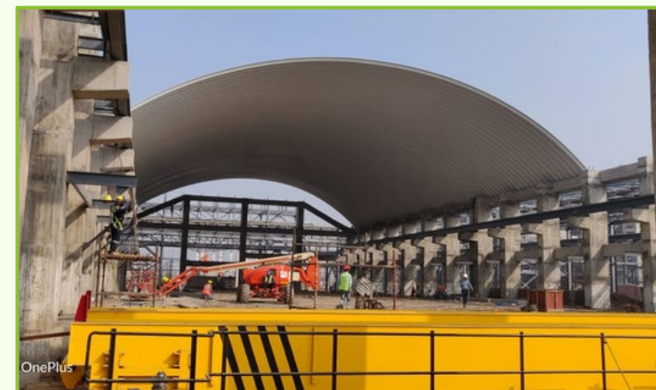
CAUSTIC SODA PLANT - DAHEJ , GUJ ARAT
